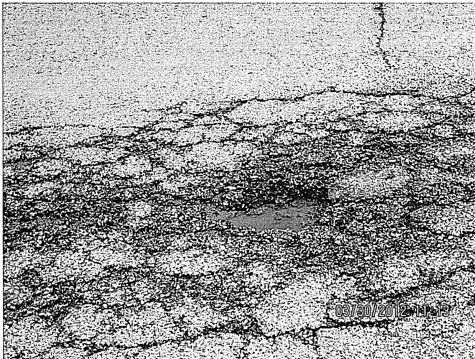
Dugan Road: Existing Pavement Conditions
