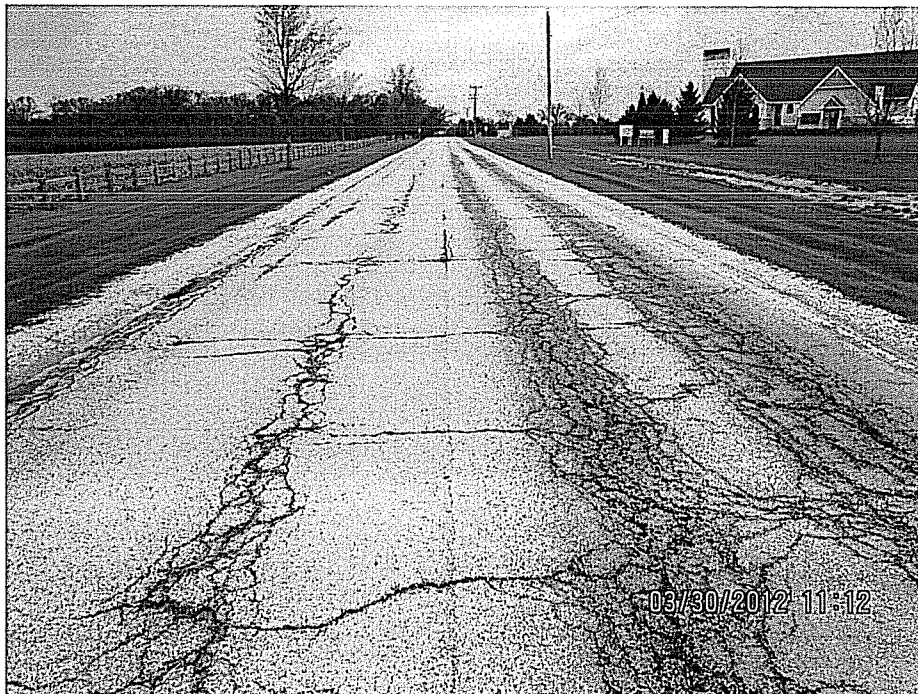
Dugan Road: Existing Pavement Conditions
