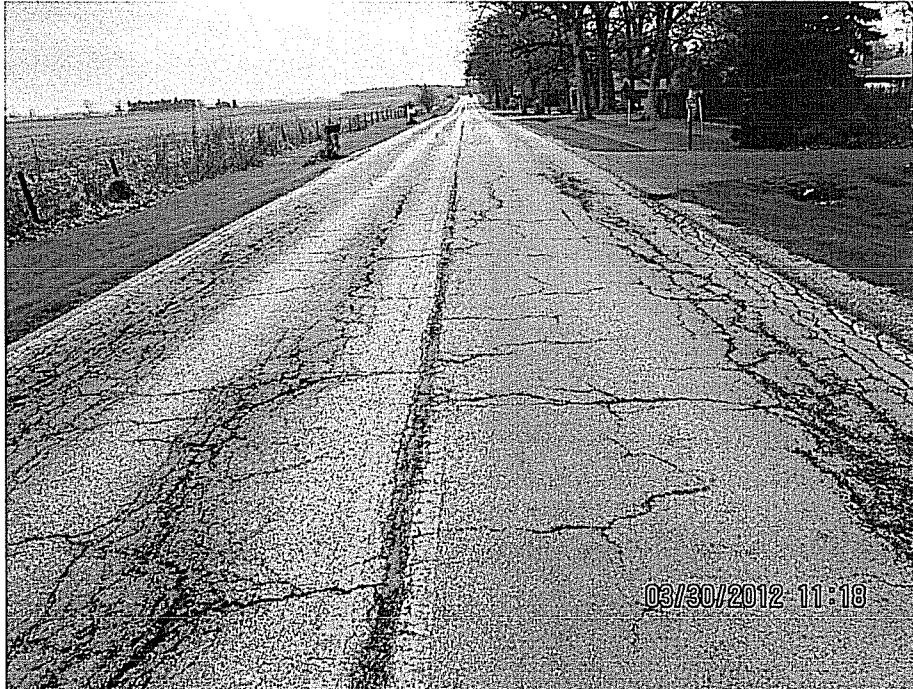
Dugan Road: Existing Pavement Conditions
